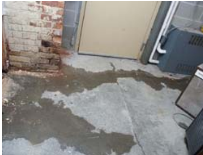
Figure 7: Regular drainage problems in the electrical room (next to the Vault).
